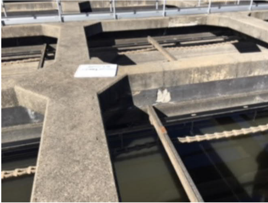
Sample #11 @ Primary Settling Tank
