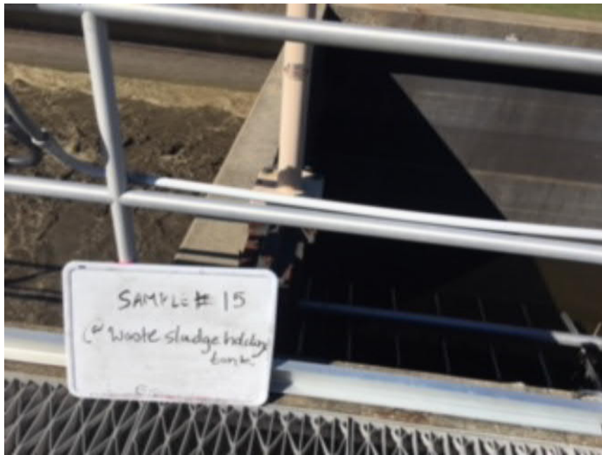
Sample #15 @ Waste Sludge Holding Tank
