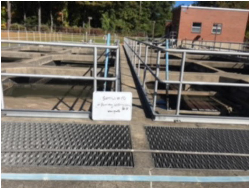
Sample #10 @ Primary Settling Tank Number 3
