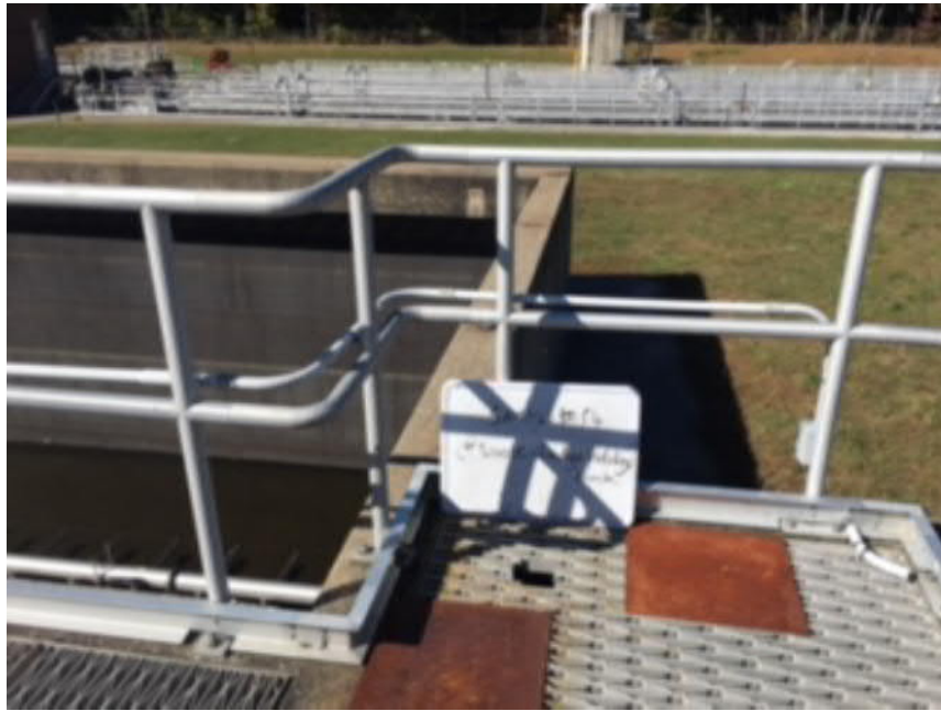
Sample #14 @ Waste Sludge Holding Tank
