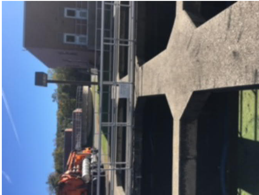
Sample #5 @ Final Settling Tank Number 2
