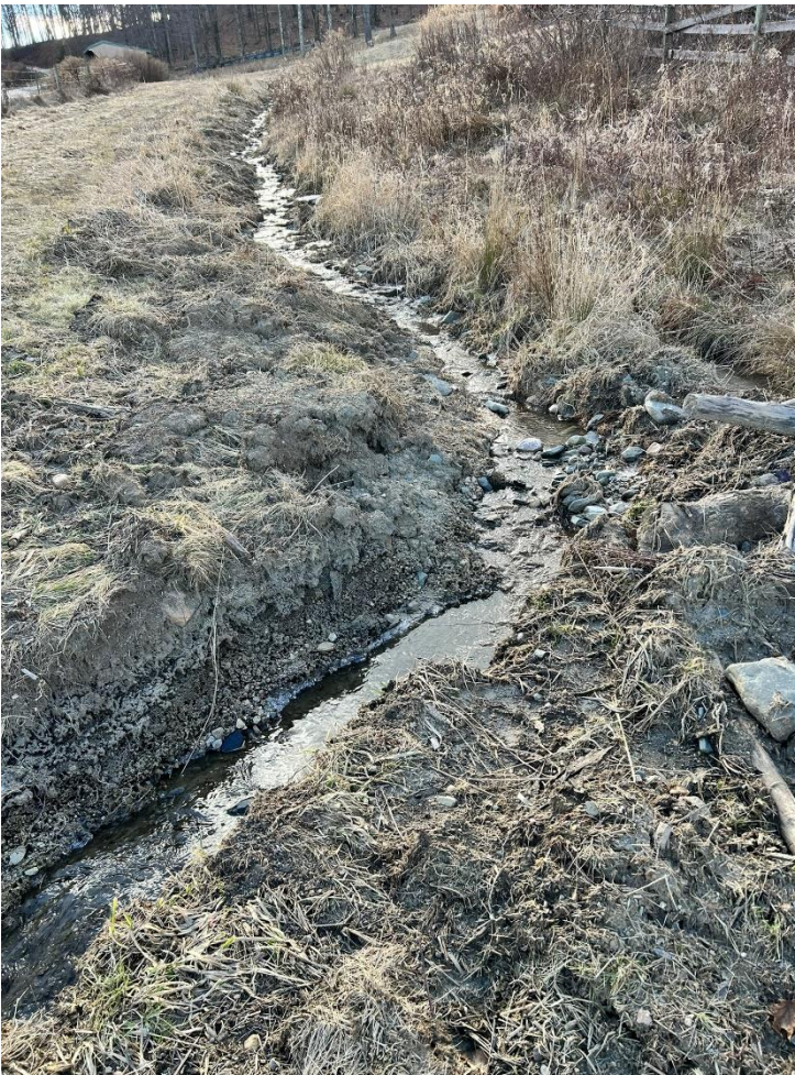
New diversion swale cut into uplands, lower portion of photo. Debris dam placed in old drainage swale, lower right portion of photo.
