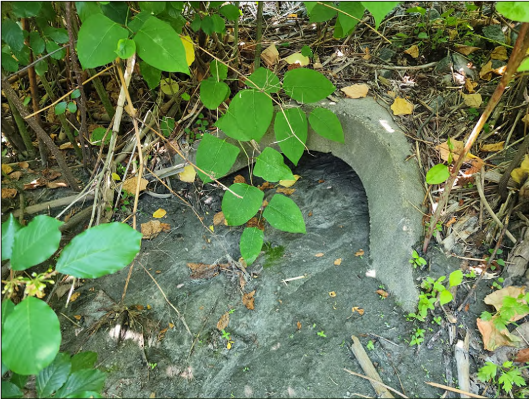
Photo 2: Mostly filled-in culvert under Winsted Road and linear park, that has brought very fine stone dust tailings to riparian wetland; facing westerly
